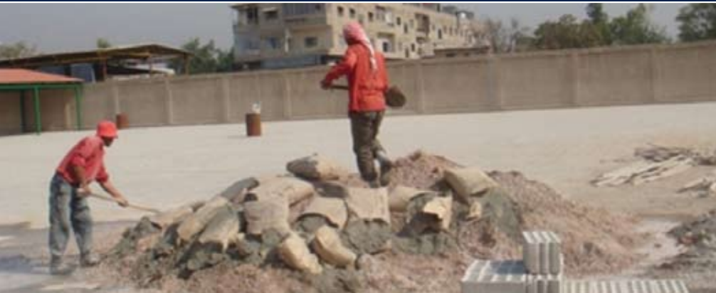
Preparatory works for building an additional classroom in the yard of Saleem Saloom secondary school
